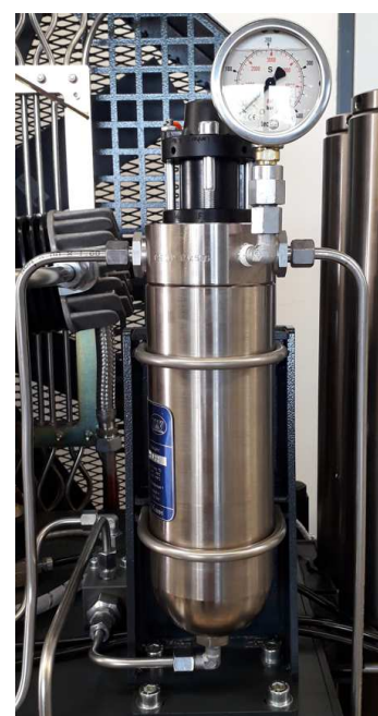
Oil / water separators
