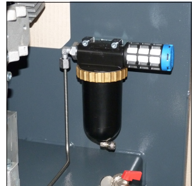
Oil / water separators final stage
