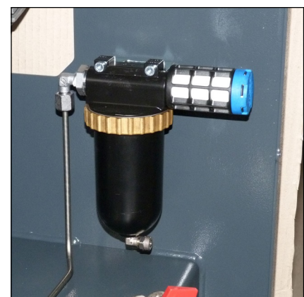
Oil / water separators final stage
