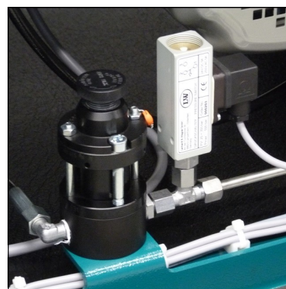
Final pressure switch
