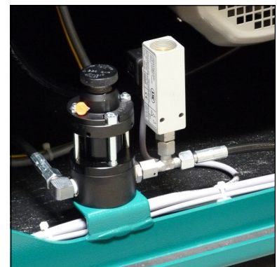
Safety valve 3rd stage
