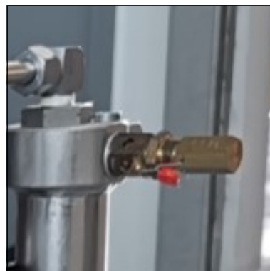
Safety valve 2nd stage
