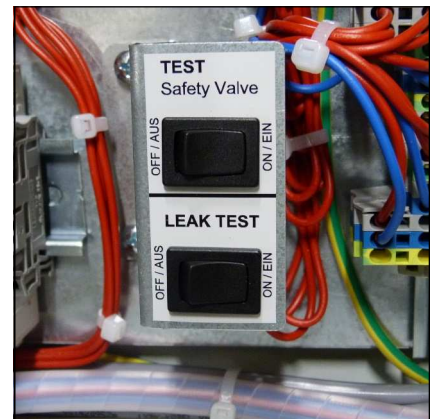
Leak test switch (lower)
