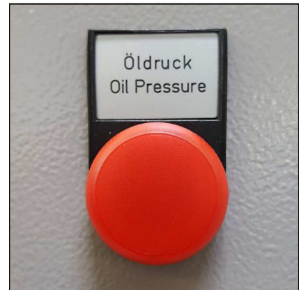
Oil Pressure Monitoring
