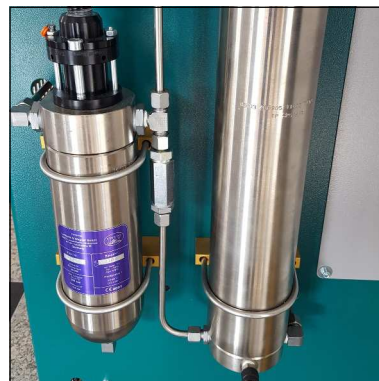
Fig. 3 - Loose pipe connections and nuts
