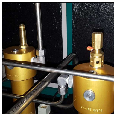
Safety valve 2nd and 3rd stage
