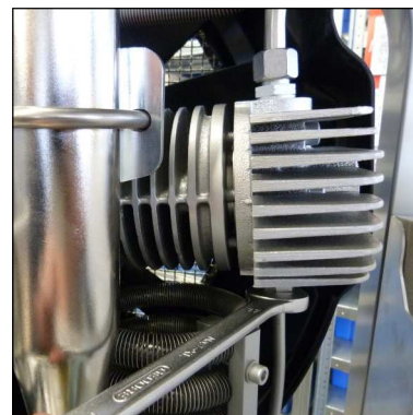
Fig. 1 - Loosen pipe connections
