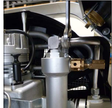
Fig. 1 - Loosen pipe connections
