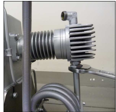
Fig. 4 - Loosen pipe connections
