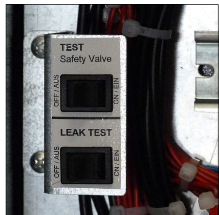
Leak test switch (lower)
