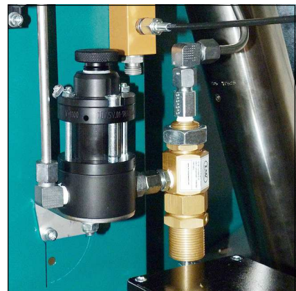
Fig. Safety valve: 225 bar (left), pressure reducer: 330 / 225 bar (right)
