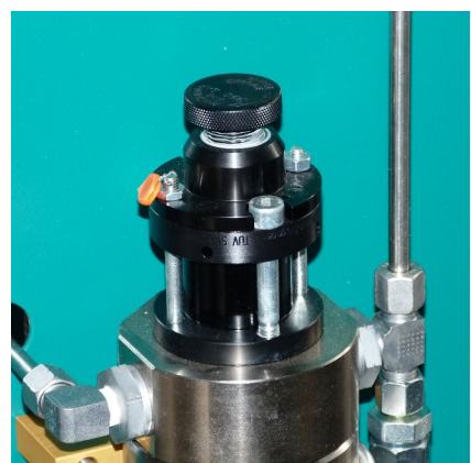
Safety valve 3rd stage
