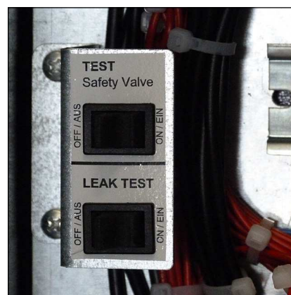
Safety valve test switch (up)
