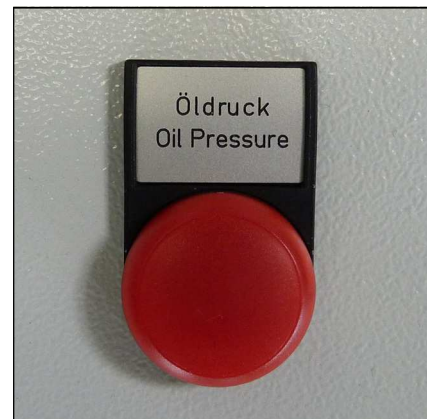
Oil Pressure Monitoring
