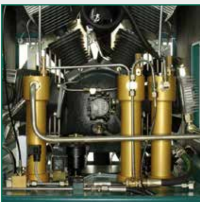
Water separators after each stage
