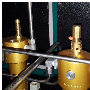
Safety valve 2nd and 3rd stage
