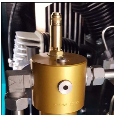
Safety valve 1st stage
