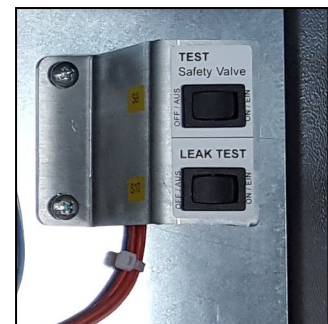
Leak test switch (down)
