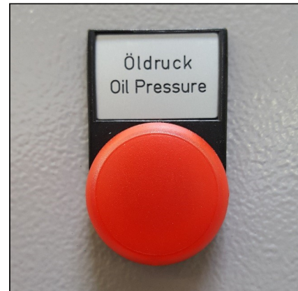
Oil Pressure Monitoring
