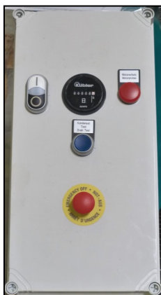
Condensate Test Drain Button
