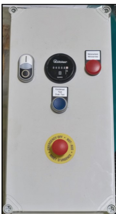
Condensate Test Drain Button
