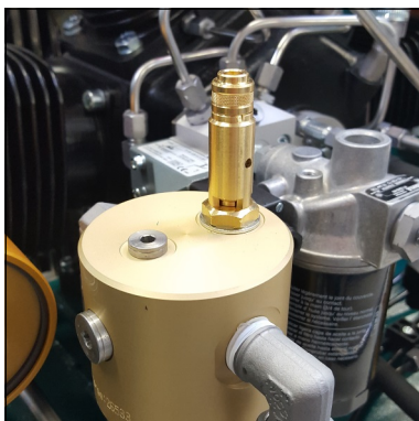
Safety valve 1st stage
