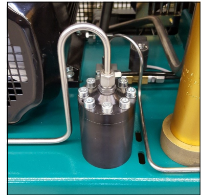
Fig. 1 - Condensate stop valve housing
