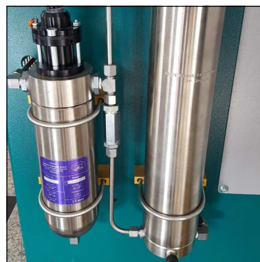
Fig. 3 - Loose pipe connections and nuts
