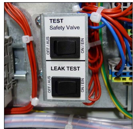
Safety Valve Test Switch (up)
