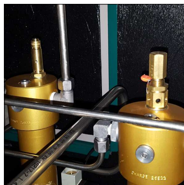
Safety valve 2nd and 3rd stage
