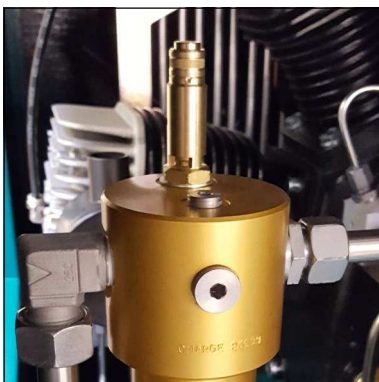
Safety valve 1st stage
