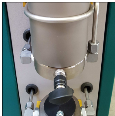
Fig. 3 - Loose pipe connections and nuts
