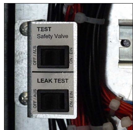
Safety valve test switch (up)
