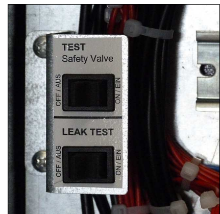
Leak test switch (lower)
