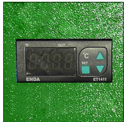
Oil Pressure Monitoring
