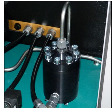
Fig. 1 - Condensate stop valve housing
