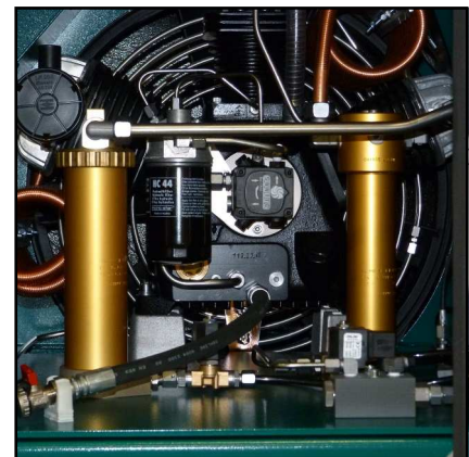
Oil / water separators 1st and 2nd stage
