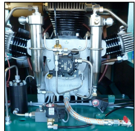
Oil / water separators 1st and 2nd stage
