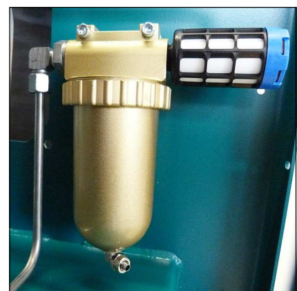
Oil / water separators final stage
