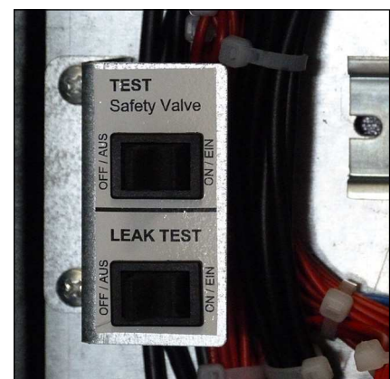
Leak test switch (lower)
