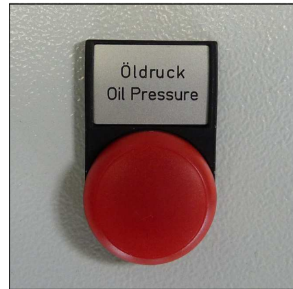
Oil Pressure Monitoring
