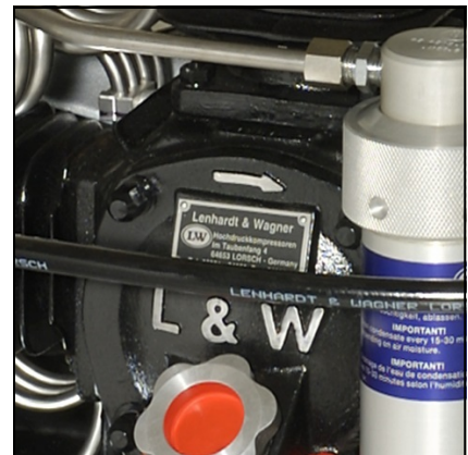
Rotation direction arrow on the compressor block
