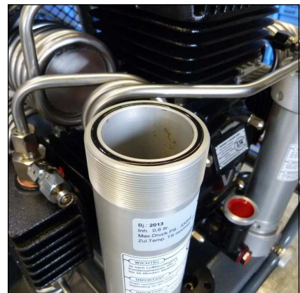
Fig. 2 - Filter housing without filter cover
