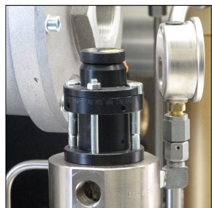
Safety valve 4th stage
