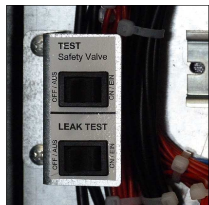
Safety valve test switch (up)
