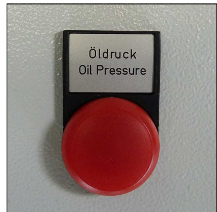
Oil Pressure Monitoring
