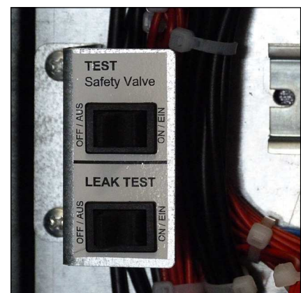
Safety valve test switch (up)
