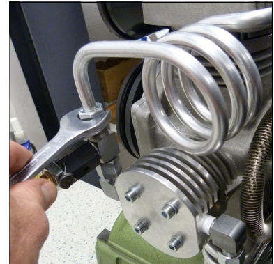
Fig. 1 - Loosen pipe connections
